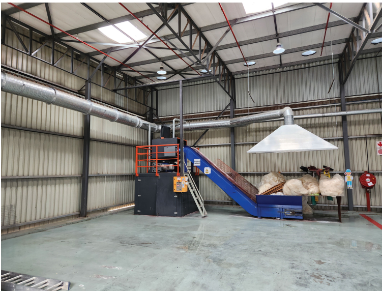
Complete extraction and ducting system installed for shredder fume capture and airflow management.
