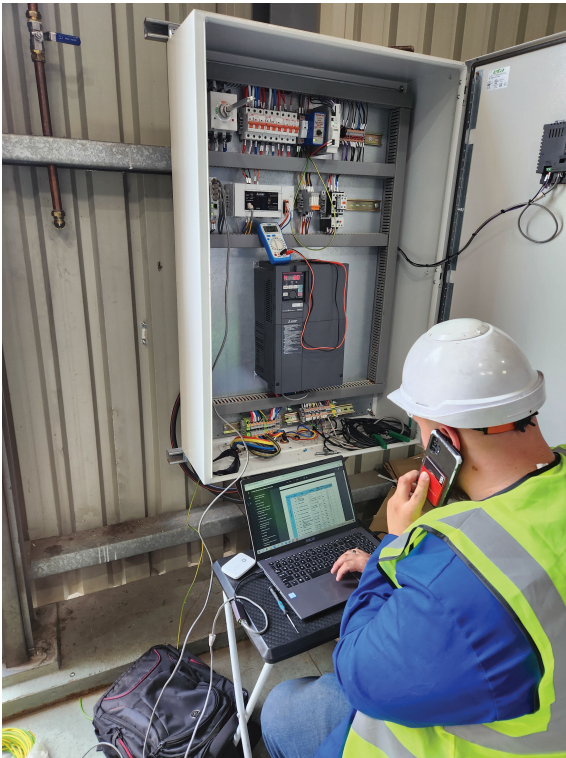
Control panel commissioning and VSD parameter configuration performed during final system startup.
