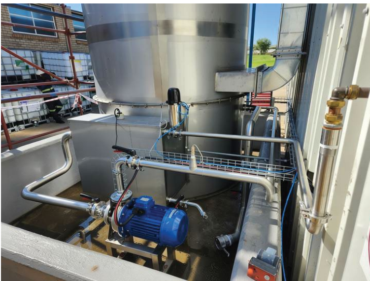
Reticulation pump and circulation system supporting continuous scrubber operation and contaminant treatment.
