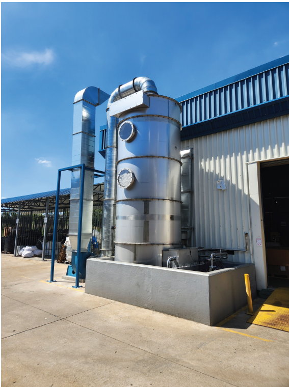
Complete industrial wet scrubber system designed and commissioned for hazardous fume extraction and treatment.
