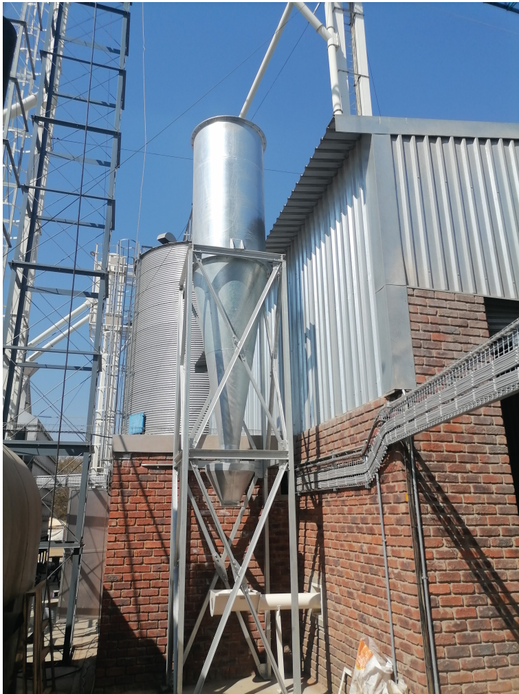
DECY Cyclone installation providing dust separation and product recovery within a grain cleaning operation.
