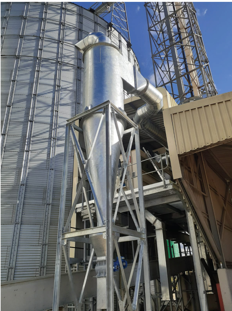
Integrated cyclone and ducting arrangement designed for efficient dust capture and airflow management.
