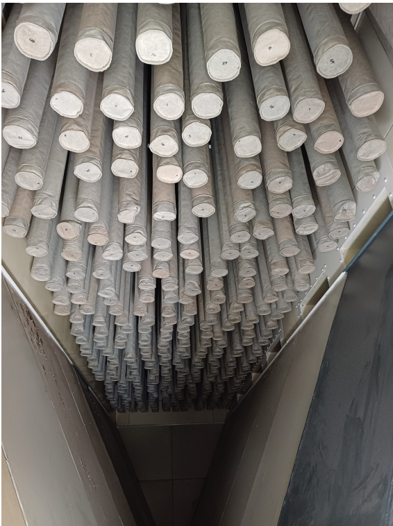
Internal view of the baghouse filtration system showing installed high-performance filter bags.
