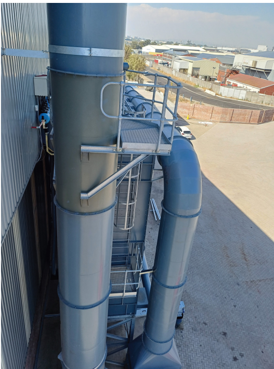
Primary fume extraction ducting and access platforms servicing the galvanizing enclosure.
