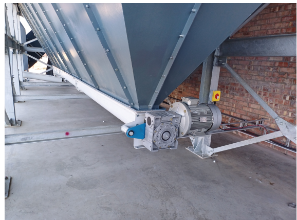
High-velocity ducting designed to maintain particulate transport and prevent condensation.
