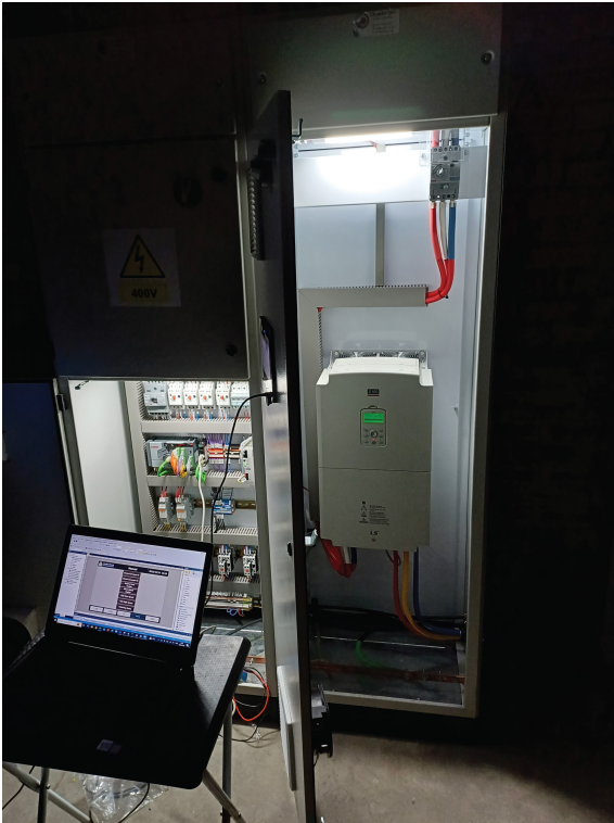
Dueltron Automation Systems (DAS) control panel incorporating PLC and VSD control.
